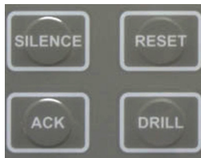
Figure 68. Control Panel Pushbuttons
