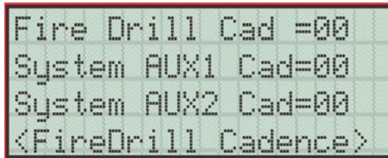
Figure 7-15 Special Cadence Patterns for Fire Drill and Auxiliary Alarm Events
